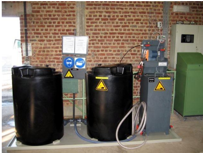
For municipal water, GO 2 TM concentrate is pumped from 1,000 liter tanks into the drinking water system. No dangerous generators or specially secured area's are necessary.
